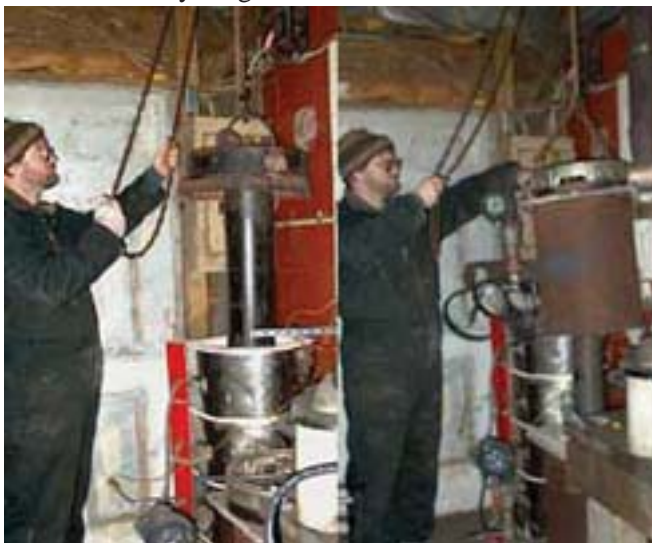
Reassembling the salt tanks once the repair and the long blade tank modification had been completed
